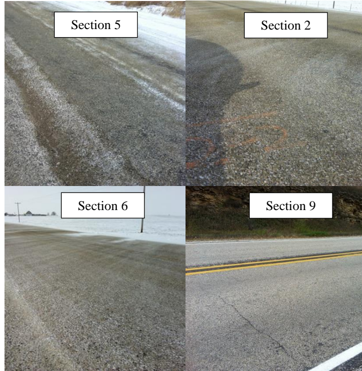
Figure 4.5. Surface Condition of Chip Seals
